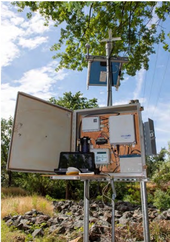
Figure 3. A view of the station house for the newly installed North Honcut Stream Gage on Honcut Creek in Butte County.
