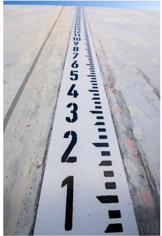
Figure 2. Several staff gauges have been installed on the inside walls of the newly constructed Lake Oroville main spillway in Butte County.
