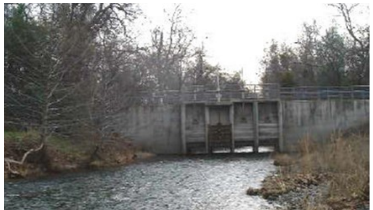
Figure 4: Box culverts regulating flow on Big Chico Creek into Lindo Channel
