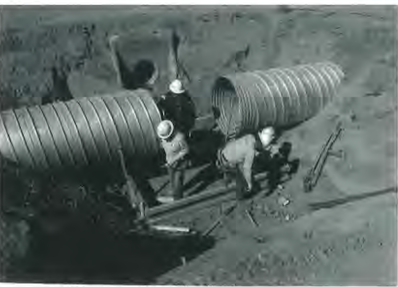
An EBID crew at work on a piping project west of Las Cruces.
