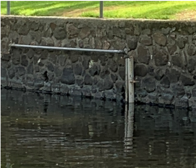
Photograph 2. Stilling well and staff gauge installed in Big Chico Creek near the 5-mile recreation area.
