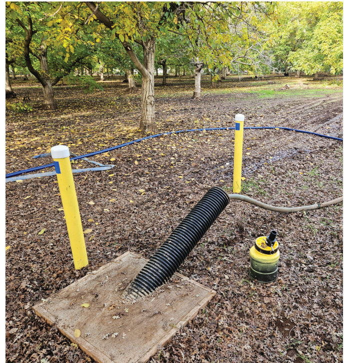
Photograph 1. Discharge line from irrigation well going into tile drain.
